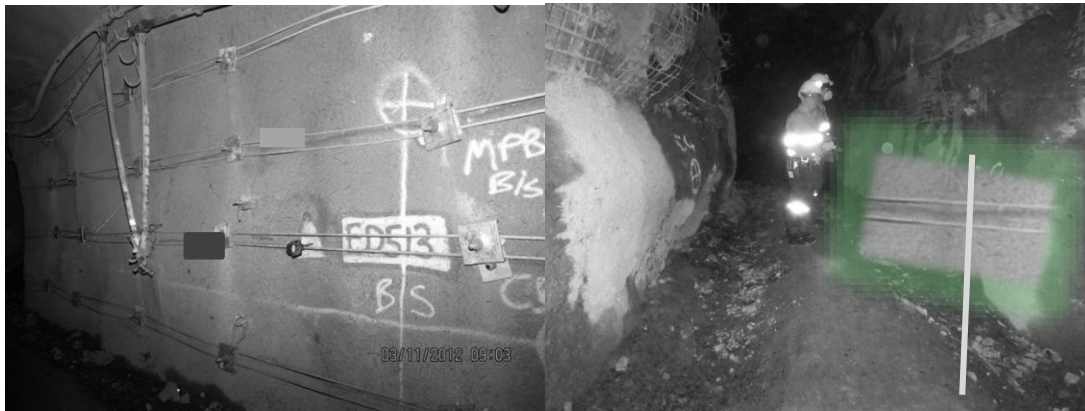
Fig. 16 JTech bolt and surface support for squeezing ground.
