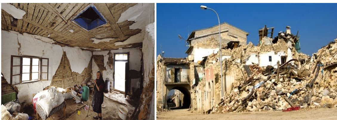
Fig. 12 Earthquake consequences in the villages accommodating the traditionally built old houses in vicinity of Mionica in Serbia.
