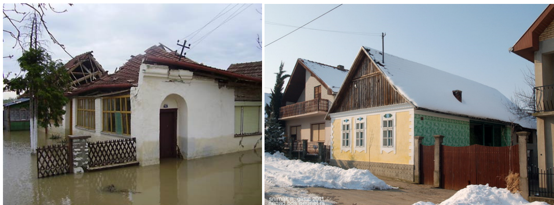
Fig. 11 Floods and constant rising damp in the village in the southern Banat as a result of the construction of a dam on the Danube river.
