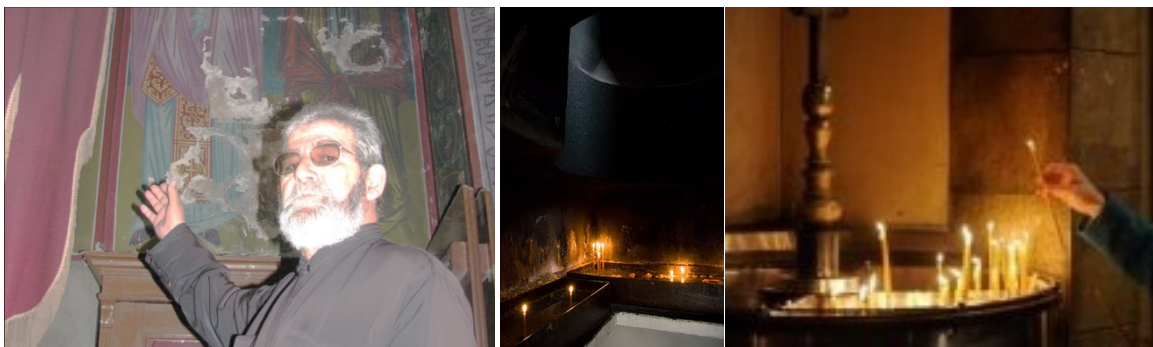
Fig. 9 Vandalism—frescoes threatened by leaking caused by theft of copper roofing and wall paintings destroyed by burning candles.
