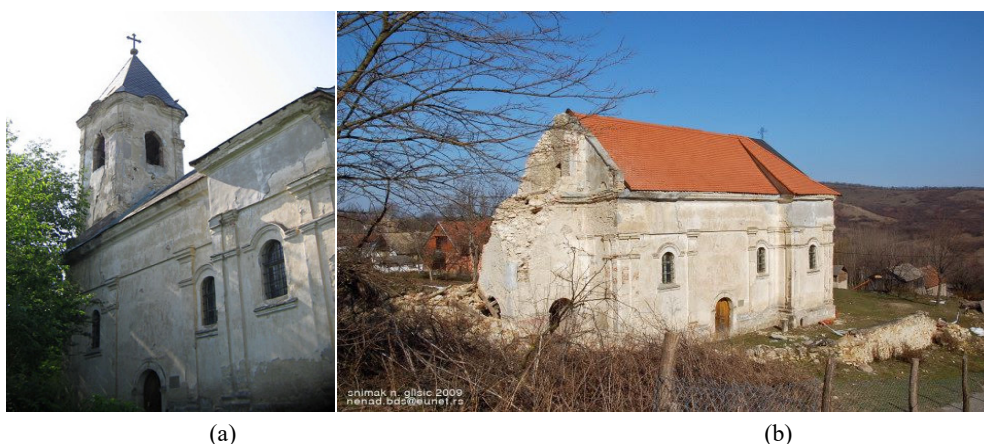
Fig. 1 (a) Church in Grabovo; (b) the bell tower was destroyed by stormy wind in 2009.
