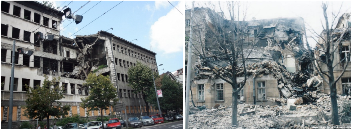
Fig. 8 One of the buildings of the Ministry of Internal Affairs of Serbia and the barracks in Zemun were destroyed by NATO (North Atlantic Treaty Organization) bombing in 1999.
