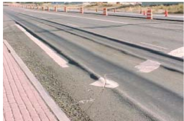
Fig. 1 Severe mix rutting.
