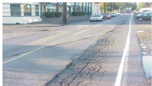
Fig. 3 Outside wheelpath rutting
