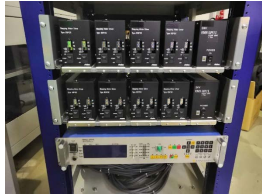
Fig. 4 Integrated controller and drive cabinet.
