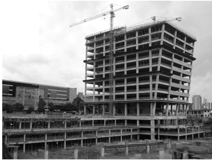
Fig. 7 Overview of the execution of the facades. Source: Archive and photo of STAMP supplied to the author, 2016.
