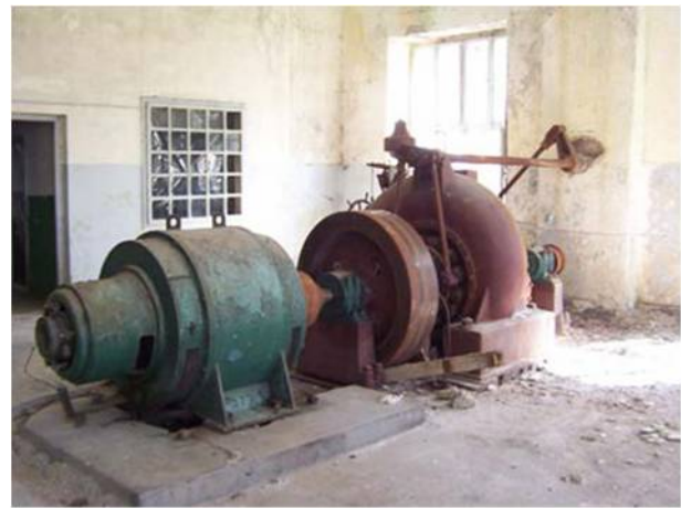
Fig. 10 Turbine out of function.
