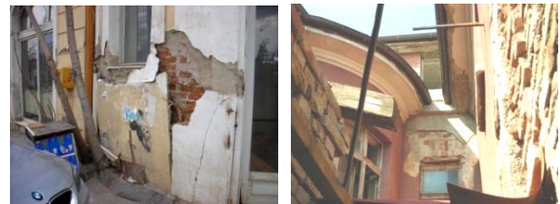
Fig. 5 The views of the building while the diagnostic phase took place in order to prepare the rehabilitation plan.
