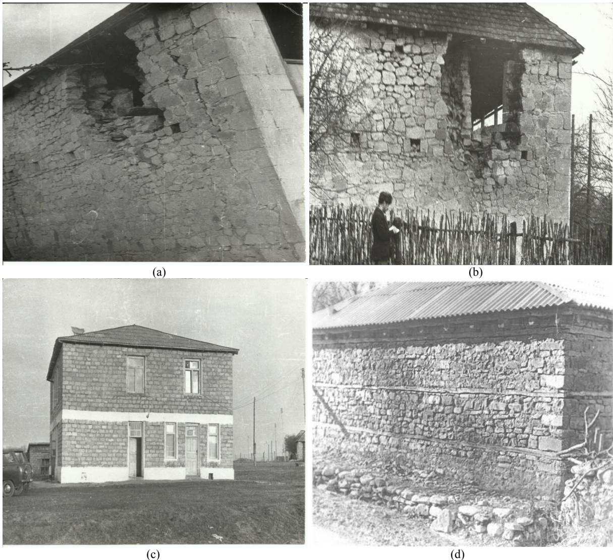
Fig. 1 Damaged buildings in the 1981 Ismayılı (Azerbaijan) earthquake: (a) Level 4 damaged building post-earthquake appearance; (b) Level 4 damaged another building; (c) Level 1-2 damaged building; (d) Level 1-2 damaged another building.
