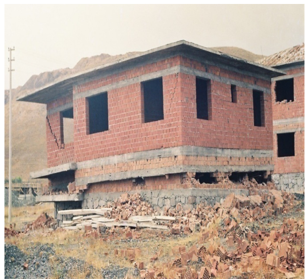
Fig. 8 Complete crushing and dissolution of the ground floor of a two-storey building with a concrete beam at the floor level.
