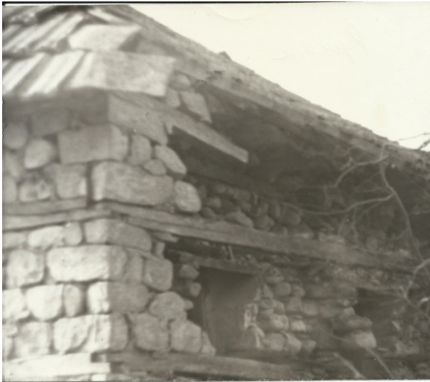
Fig. 7 A building where the distance between wooden beams is not suitable for masonry quality.
