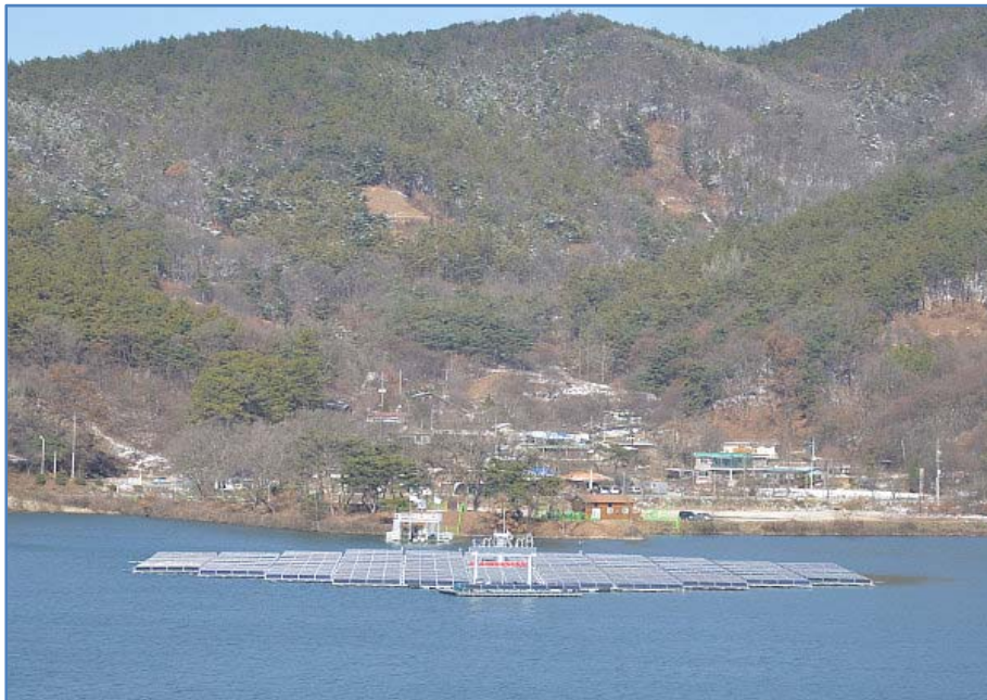
Fig. 2 Floating tracking PV system in Korea (Source: SolarPark Korea).
