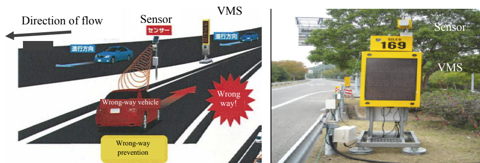
Fig. 1 Roadside wrong-way warning systems with different types of sensors.
