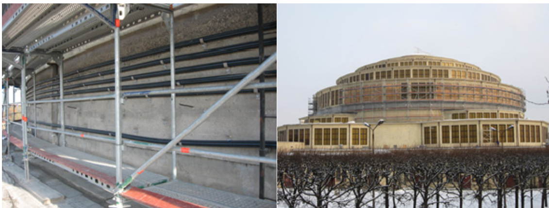
Fig. 3 Reinforcement of the lower extended rim—arrangement of cables and securing of the mortar (photographer: R. Dzugaj).
