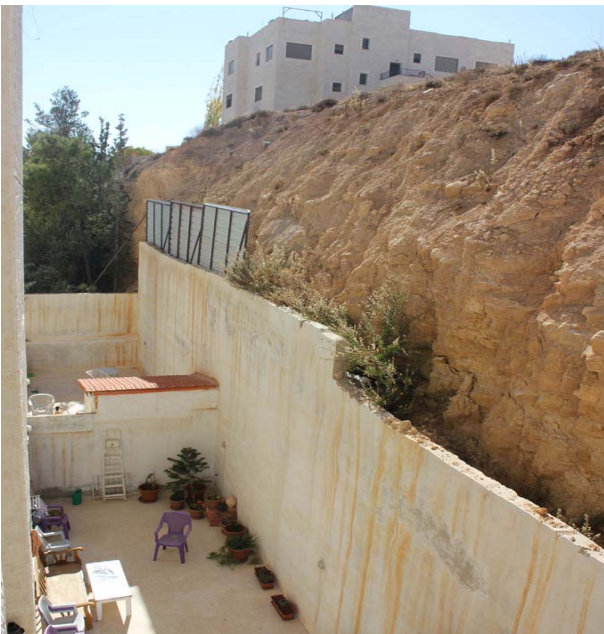
Fig. 10 Retaining walls on severely cut slopes.
