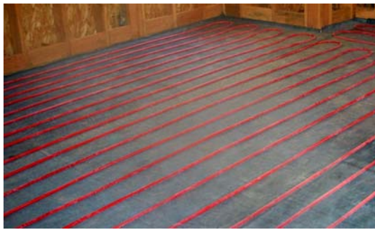
Fig. 8 Aerogel blanket used under heating pipe.
