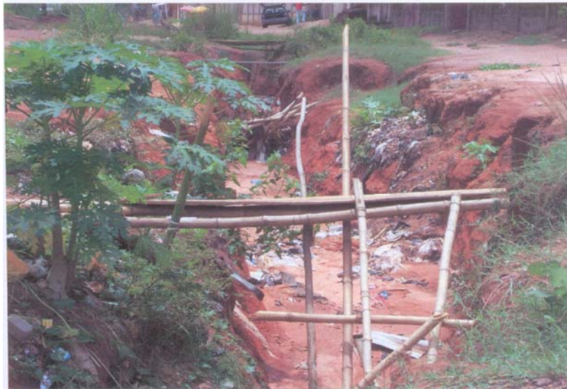
Fig. 5 Ikenegbu road in Owerri destroyed by gully erosion.
