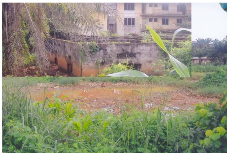
Fig. 6 Abandoned building in Umuna Orlu due to seasonal floods.
