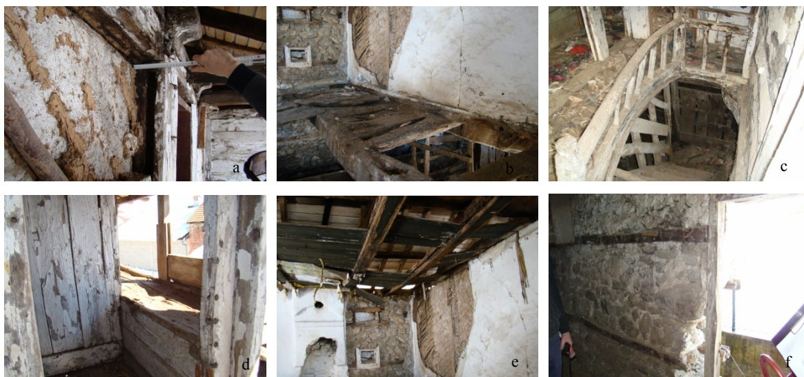
Figure 2. a. Damaged internal wall constructed by clay reinforced with timber willows; b., c., and e. deterioration of a timber elements at ceiling/flooring and staircase structure; d. pour maintenance of planking envelope; f. misapplied of structural conservation.
