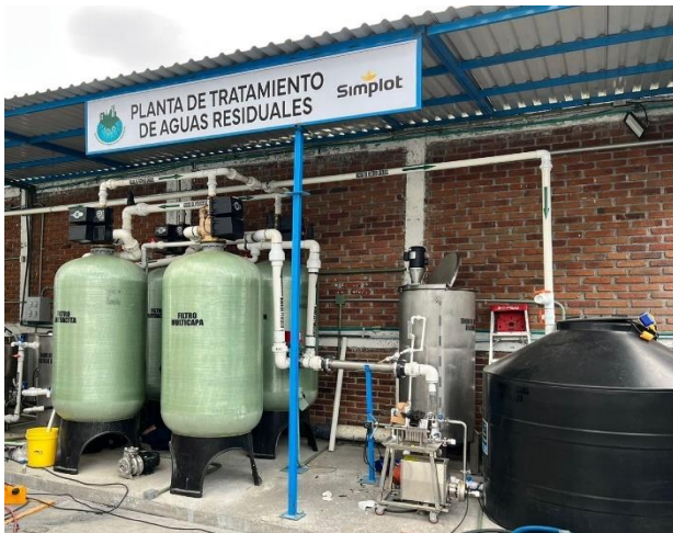
Fig. 2 Wastewater Treatment Plant.
