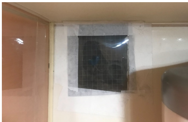
Fig. 4 Sealed vent in the bathroom of a residential apartment in Tomsk.
