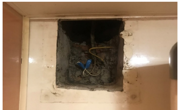
Fig. 3 The air vent in the bathroom of a residential apartment in Tomsk without a fan.
