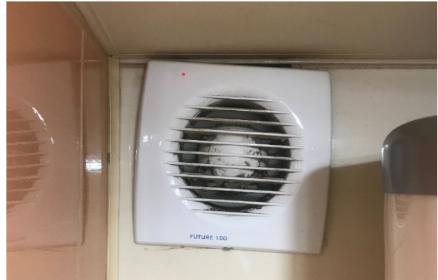
Fig. 1 Wall fan installed in the toilet of an apartment on the 3rd floor of a 9-story building in Tomsk.
