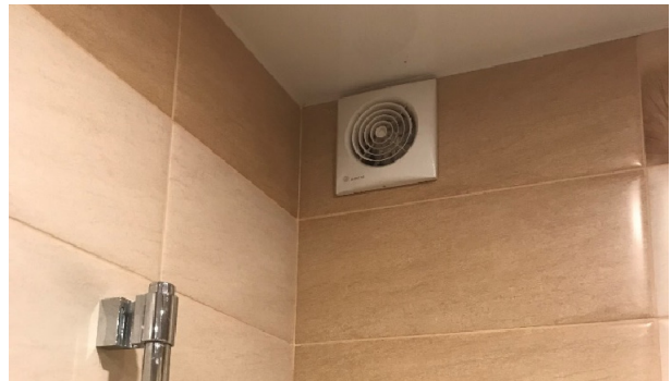
Fig. 2 Wall fan installed in the bathroom of an apartment on the 9th floor of a 10-story building in Tomsk.
