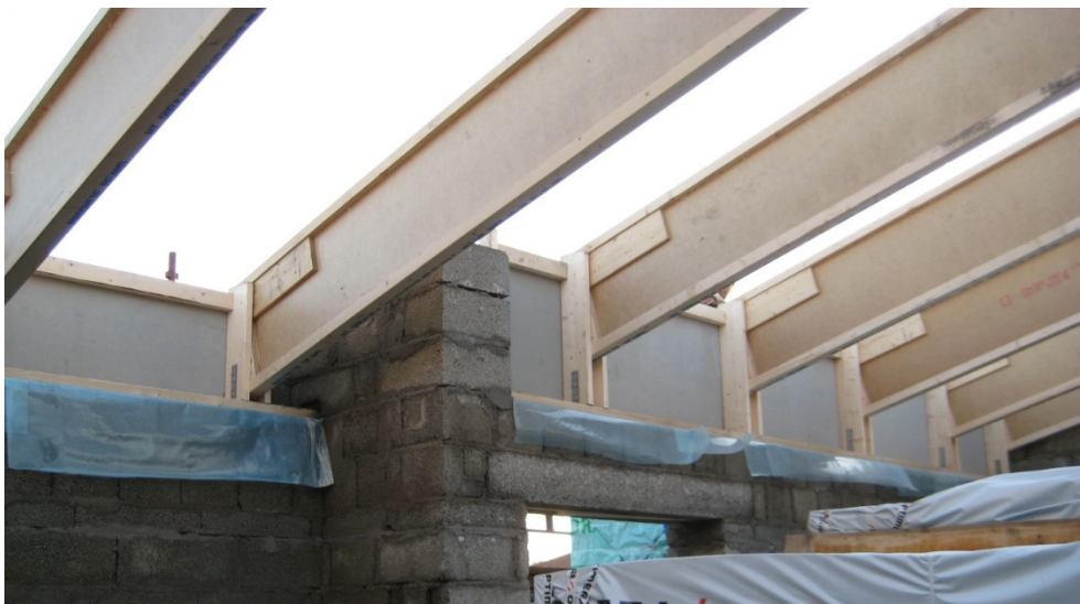
Fig. 3 Pinching of the plastic foil between top of the masonry wall and wooden beam.
