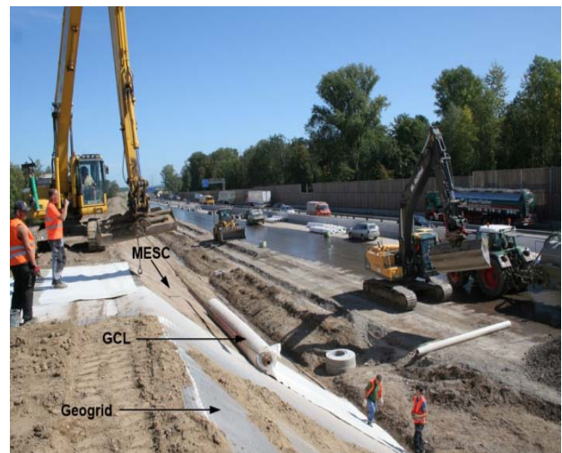
Fig. 8 Use of a geogrid reinforcement in construction method B for encapsulation of MESC on a 1:1.5 (v:h) slope for slope stabilisation.
