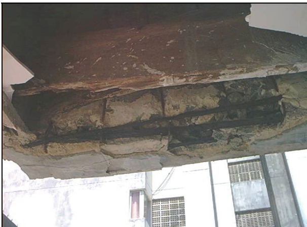
Fig. 7 Beam reinforcement corrosion with section loss in Building B.
