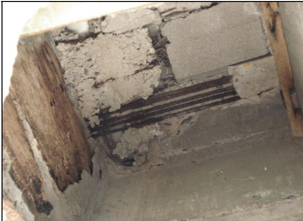
Fig. 6 Corrosion of slab reinforcement of Building A.
