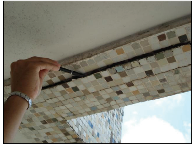
Fig. 1 Fissure in the edge beam of Building A.
