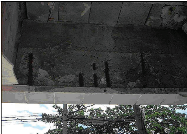
Fig. 9 Stirrup of the exposed beam, with corrosion, in Building B.
