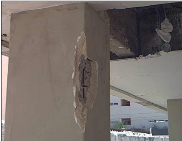
Fig. 8 Detachment column due to reinforcement corrosion.
