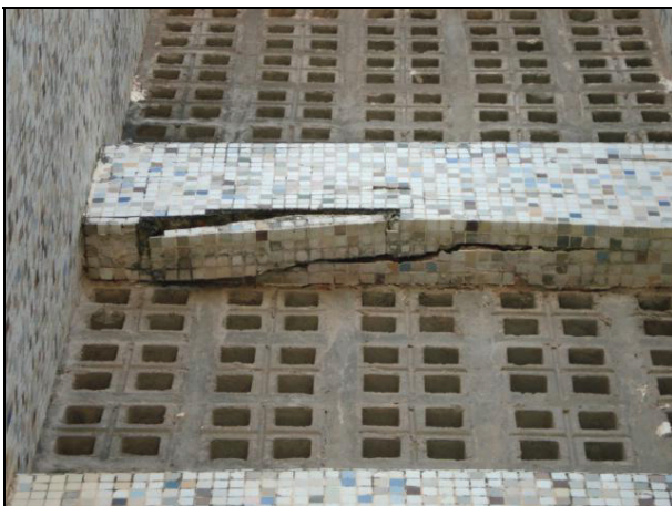
Fig. 4 Detachment of reinforced concrete beam of Building A.
