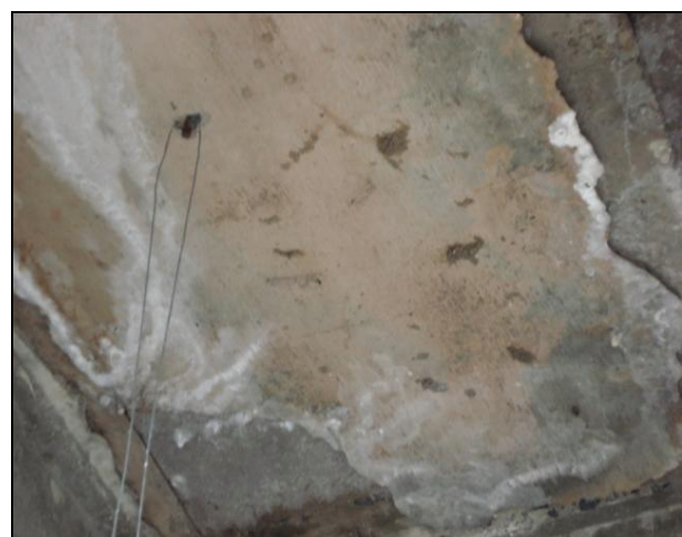
Fig. 5 Efflorescence on slab of Building A.
