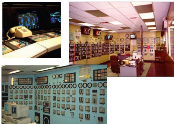
Figure 2. First generation of control room (Nimmo & Moscatelli, 2004).
